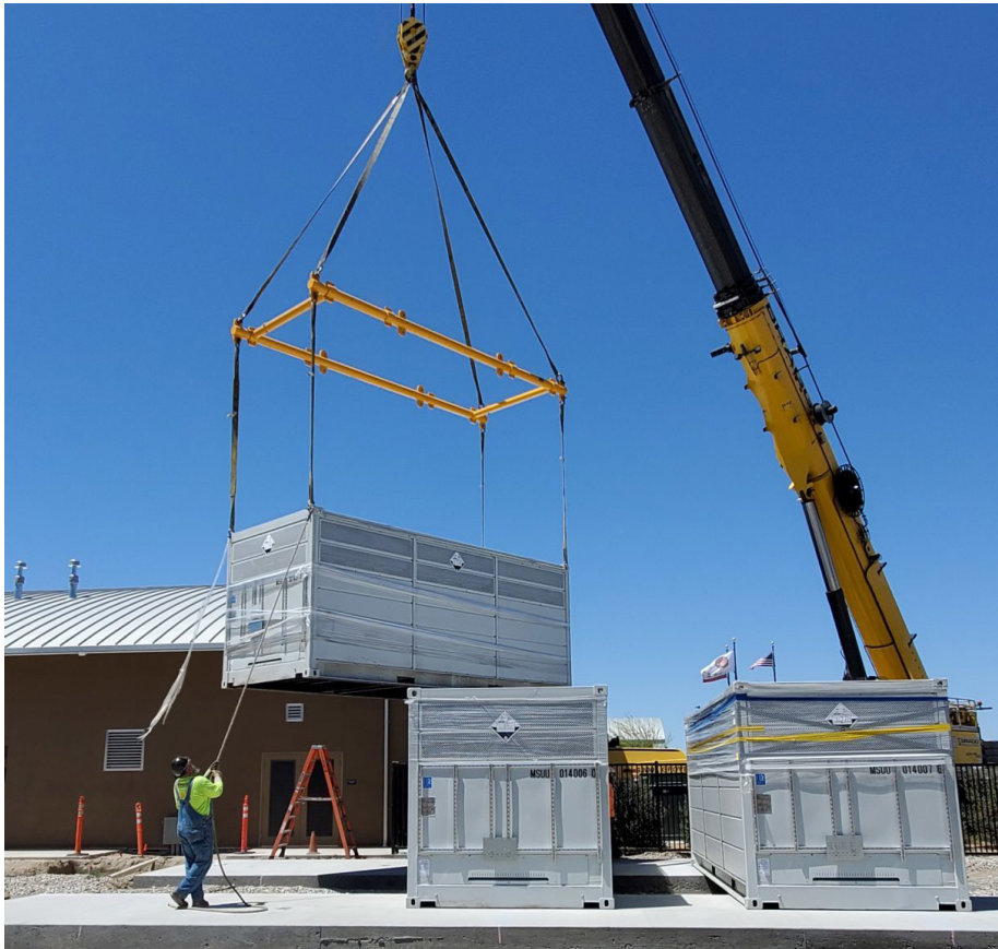
Photo courtesy of Invinity Energy Systems
