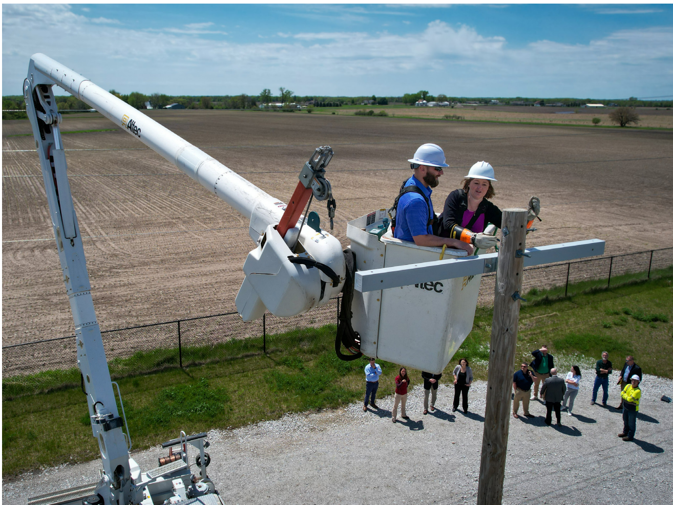
Line Supervisor Brian Killeen shows Iowa Attorney General Brenna Bird how difficult it is working in their thick electrical insulated gloves.
