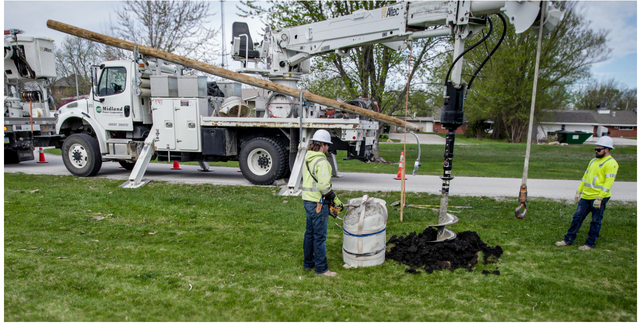
Digging deep: Linemen Wyatt Tharp and Colton Zalesak set two donated poles with attached LED security lights at the retirement center to help keep residents and visitors safe.
