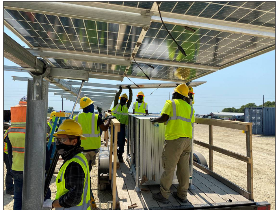
Workers from Renewable Energy Systems (RES), the installation contractors for Wapello Solar, install the bifacial panels on the single-axis tracking system. Single axis solar trackers track the sun east to west, rotating on a single point, moving either in unison, by panel row or by section.
