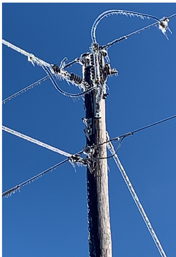
POWERING DOWN, Page 3 Ice on Midland Power lines in November 2020.
